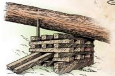
Fig 5:- Part of the weight of the remaining trunk is taken up by shims placed near the root ball.
